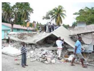
House in Jacmel after the 7.0 earthquake
